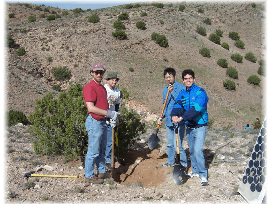
Students in the Observational Seismology course (GEOP 524) and Dr. Rick Aster, another Geophysics faculty, happily digging a hole for the installation of seismic station CAR in the Quebradas.
