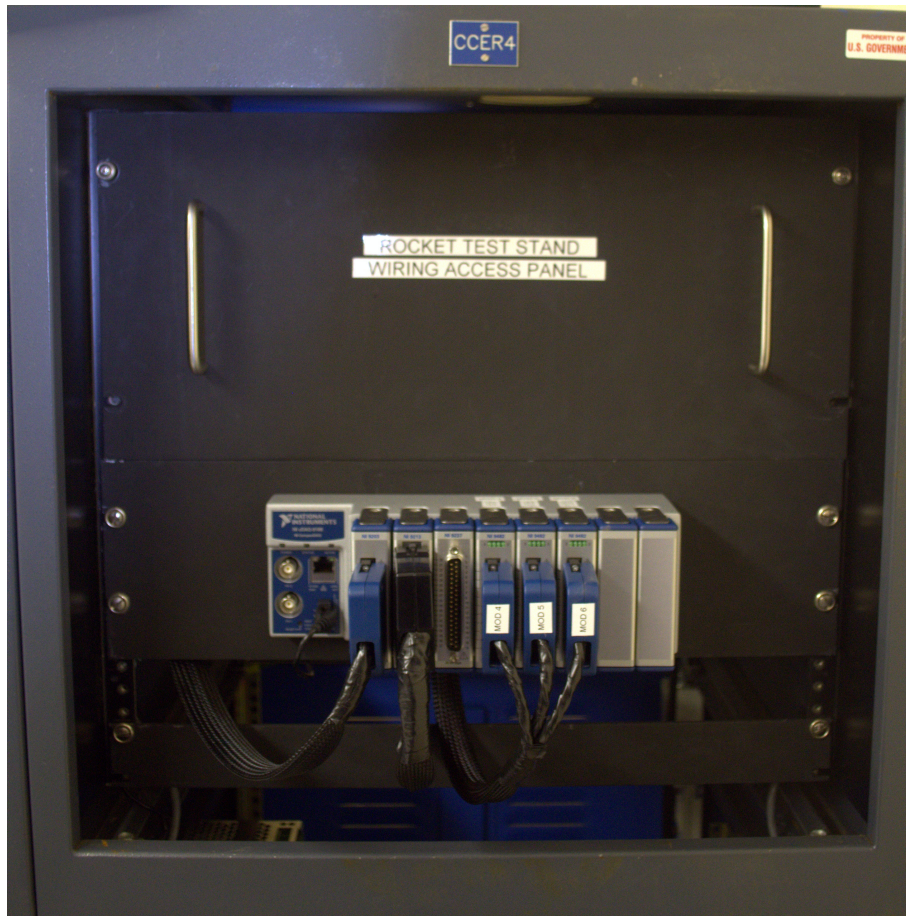
Figure 4.15: Installed cDAQ-9188 control and data acquisition system
