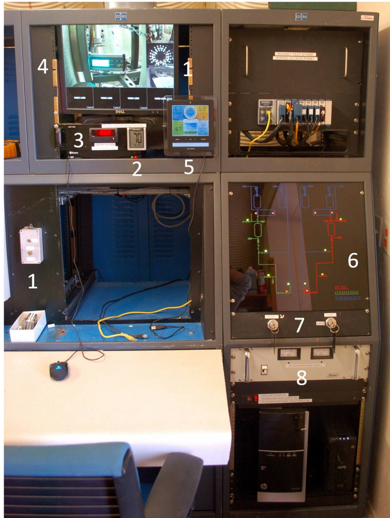
Figure 4.18: REF control console. Visible are: Deadman's switch (#1); Fuel galley temperature monitoring (#2); Igniter supply voltage (#3); Video observation system (#4); Weather station (#5); Valve status indicator panel (#6); Propellant loading controls (#7); and system power supplies (#8)
