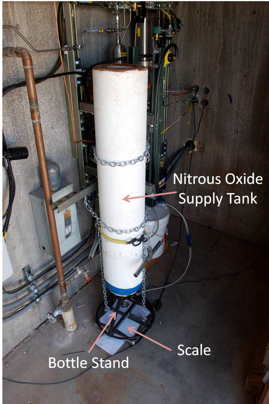
Figure 4.12: Inverted nitrous oxide source cylinder installed in fuel galley
