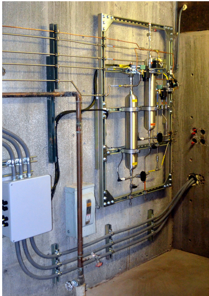
Figure 4.8: Installed propellant run tank panel
